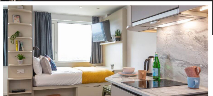
Firechief Kitchen Stove Guard installed in a Gold Studio apartment in the Vega development
